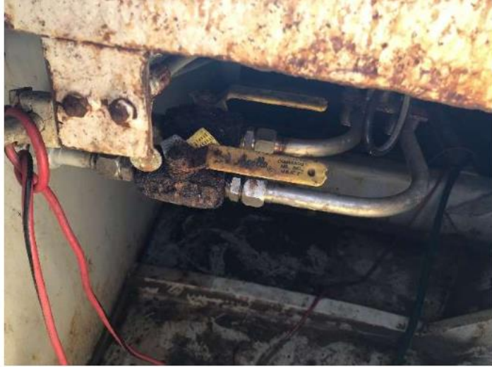
Figure 1: Corroded hydraulic steering cutoff valve, improper wiring configuration, and rusted bottom plate.
