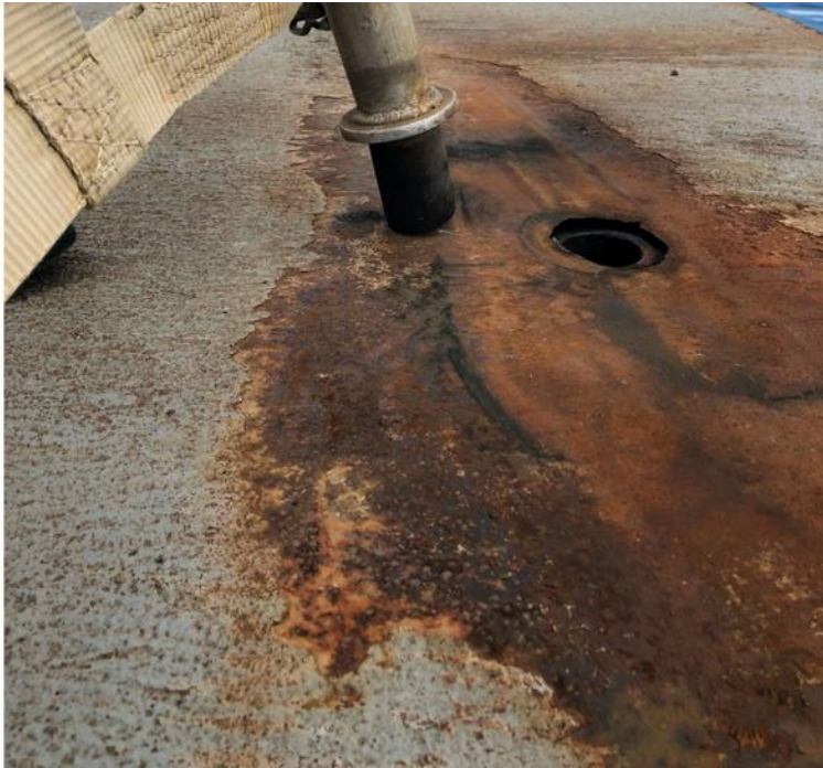
Figure 19: Stanchion system showing substantial corrosion, rust, and paint chipping.
