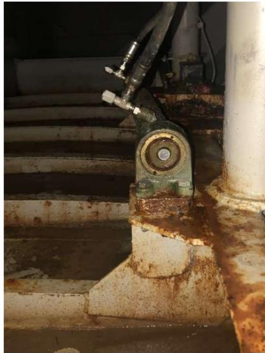
Figure 2: Corroded steering gear ram foundation and rusted bottom plated.
